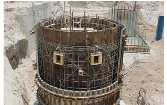
New Air Cargo Lift Station (GBIA) Houston, TX
